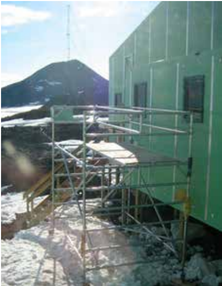
Mobile scaffolding – not the easiest ground conditions for meeting daily manoeuvrability. Photo courtesy of Linda Kestle.
