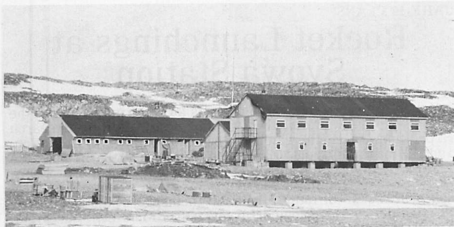
Buildings under construction in the 1976-77 season at Rothera, the new British Antarctic Survey base on Adelaide Island off the Antarctic Peninsula. The base, originally named Rothera Point, is 64km to the north-east of the old Adelaide Island base.
